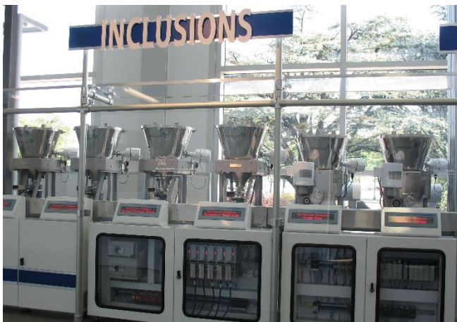
The volumetric feeders are installed side-by-side in a straight line, and a belt conveyor moves the chocolate base bars from right to left, first under two screwfeeders and then under four vibratory feeders.
