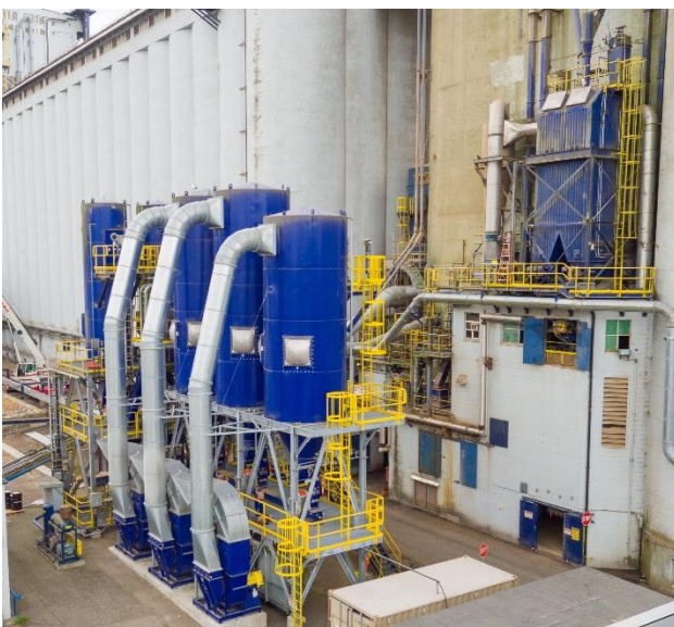
Viterra's Pacific and Cascadia terminals process a wide range of grain products, which generate a lot of dust that needs to be contained and collected.
