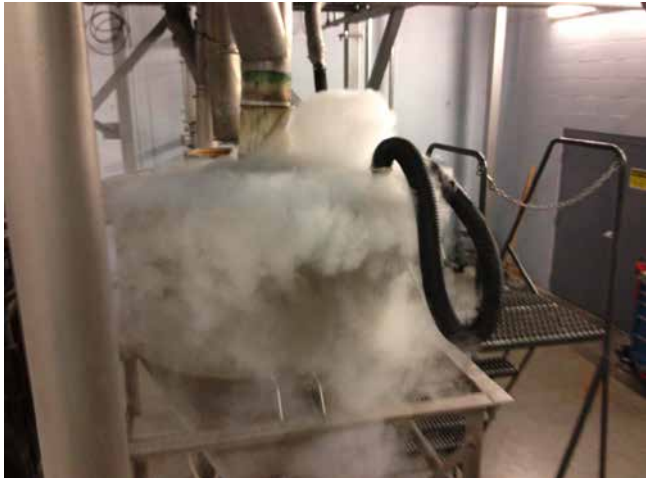
Conveying dry ice through the piping can remove build-up and deposits in the line.
