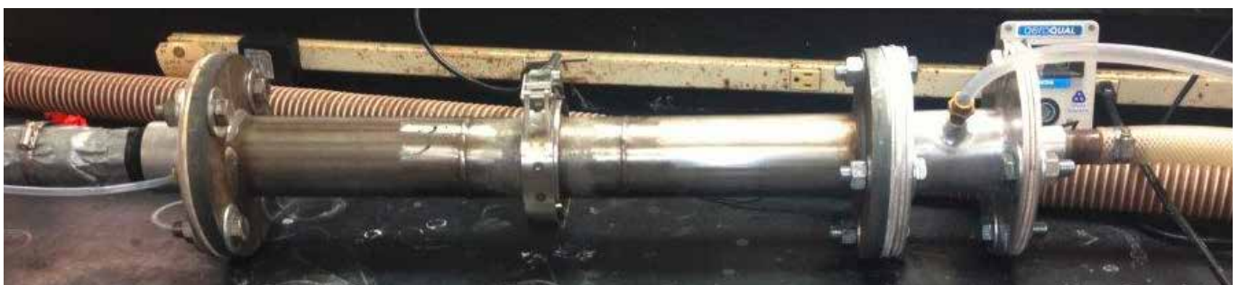
Piping used to pump ozone through lines.
