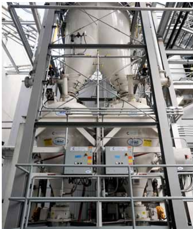
Clyde Process Twin Dense Phase CD Pumps
