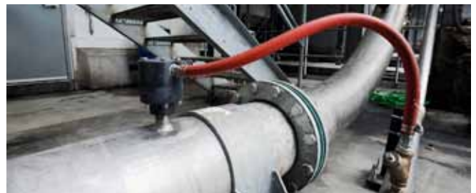
Pneumatic conveying pipeline at Imperial Sugar
