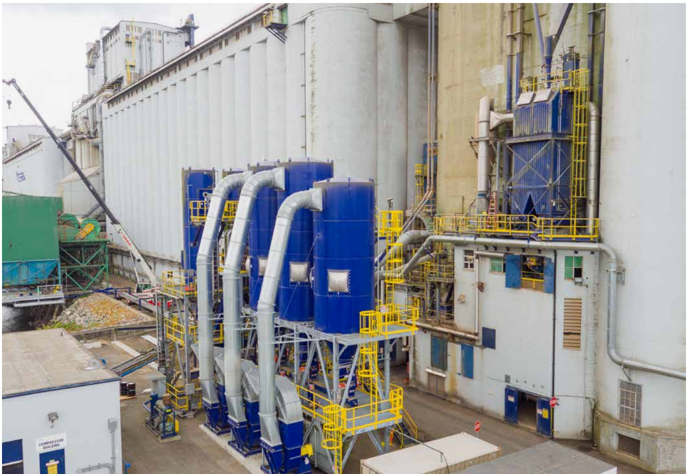
Figure 1. Viterra's Pacific and Cascadia terminals process a wide range of grain products, which generate a lot of dust that needs to be contained and collected.
