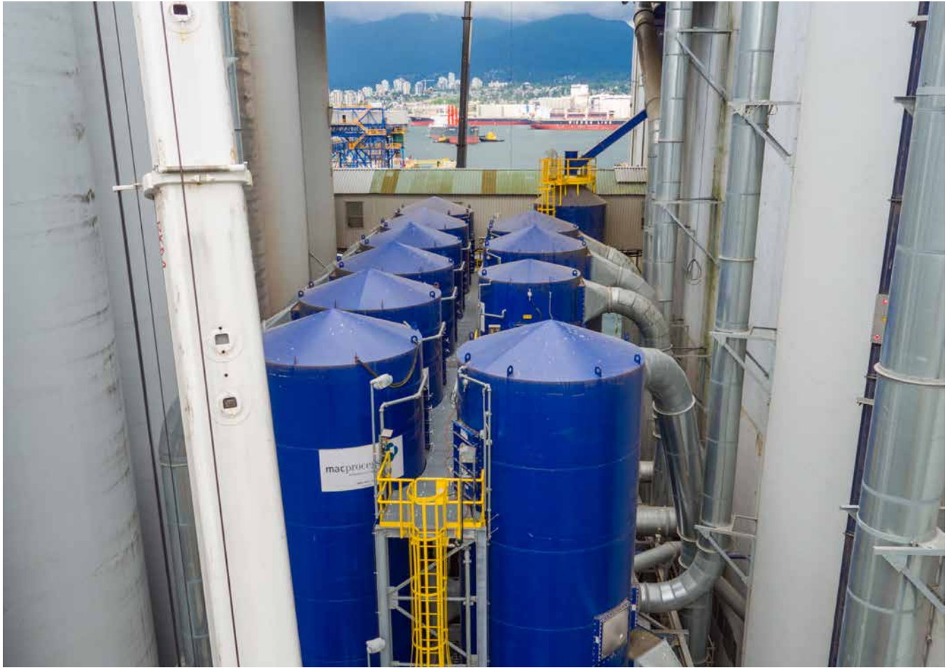
Figure 2. Viterra installed MCF PowerSaver dust collection systems at two grain processing terminals to improve their dust collection process.
