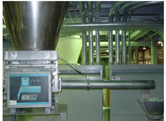
The feeder's controller monitors the hopper's load cells to ensure a continuous and accurate feedrate to the twin-screw extruder.
