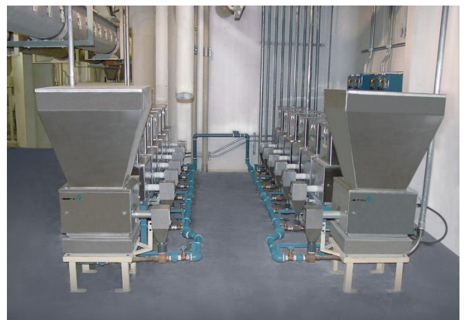
To prevent floor vibration from creating weighing errors, each feeder in this batching system rests on a scale mounted on a vibration-isolation platform.
